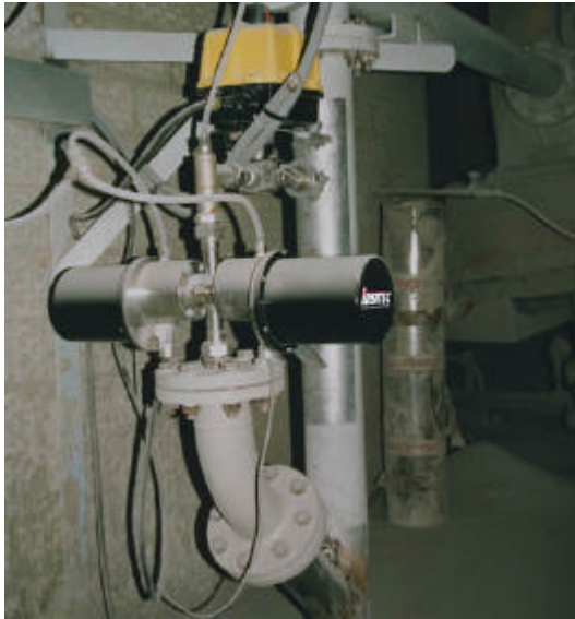
Figure 1. EPCS and interface in Cement Plant
